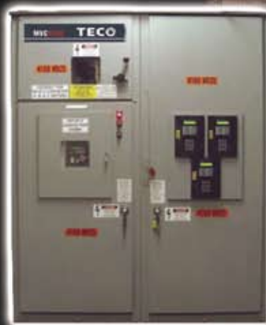
4160V, multi-motor Controller designed to simultaneously start (3) 600HP conveyor motors.
