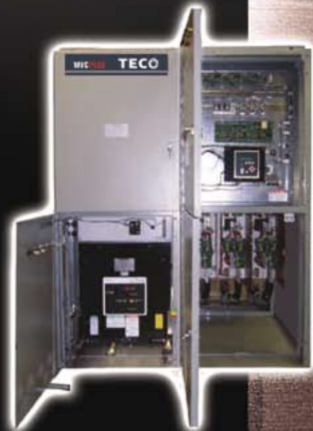
4160V, 1000A Motor Controller with Synchronous Controller for 10,000 HP gas compressor.
